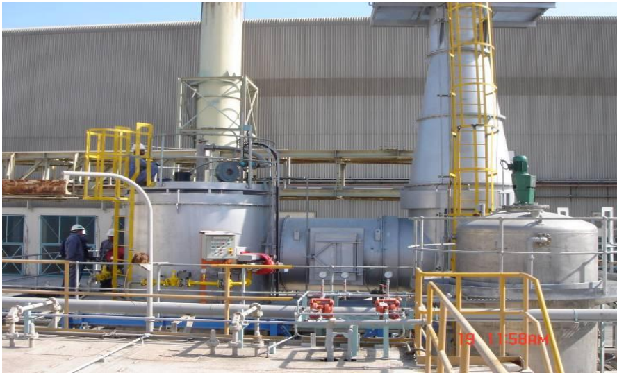
Liquid Waste TO for spent aqueous rolling mill coolant 24,000 litre/day
