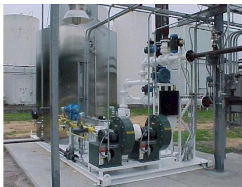
Sewage Treatment works Methane Flare system
