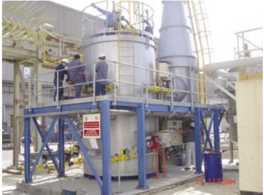
Liquid aqueous waste incinerator Khuf gas fired, 24,000m 3 /hr - Bahrain
