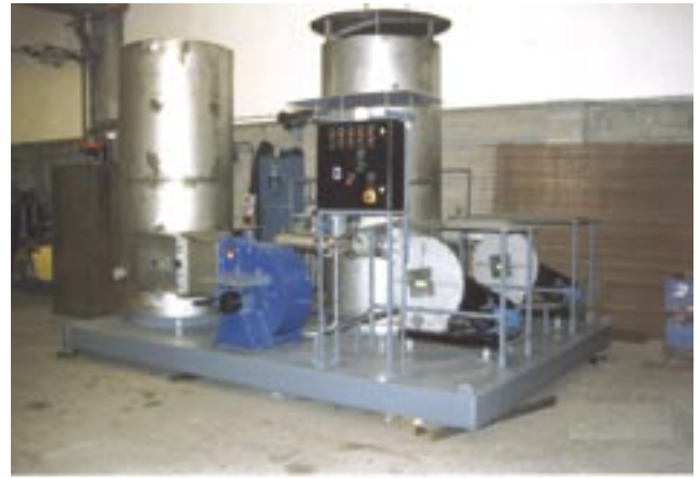
Landfill Gas Flare 5500m 3 /hr - Colombia
