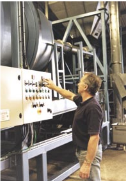
Automated PLC controls
